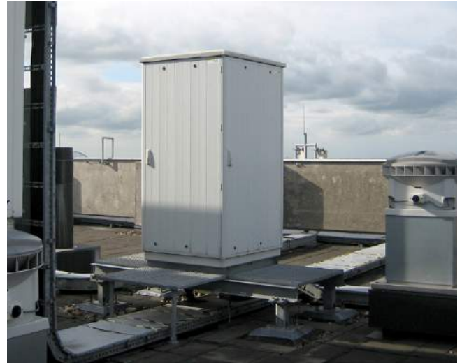
Roof mounted IP55 Outdoor UPS Cabinet
