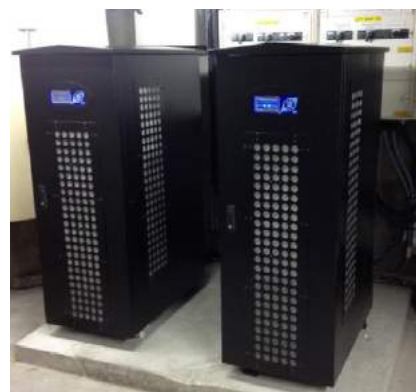
2x 80kVA High Internal Protection IP42 UPS supporting residential lifts in the UK
